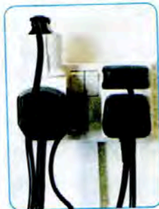
Figure 11.18 Many plugs connected to the same power point
